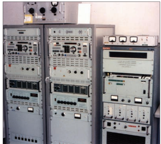
Fig. 3.1: Two Mark F six tone piccolo installation units under the antenna tuning unit for the transmitter.
